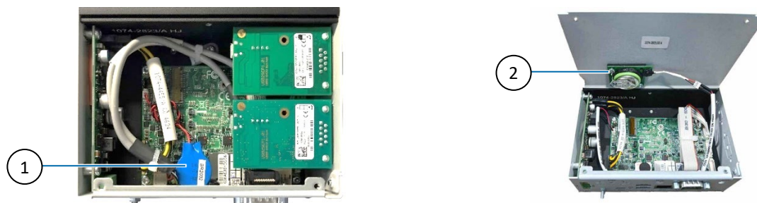
Figure 12: RTC Lithium Battery Installed
